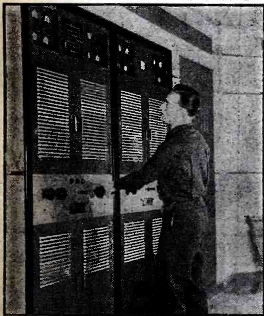
The new RCA model D-1 1,000-watt transmitter used at station CKCK, Sask., Canada. All components are enclosed in modernistic steel cabinets as shown.
